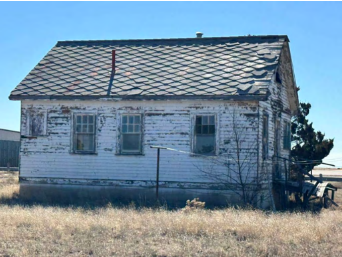
Dilapidated Housing Stock
